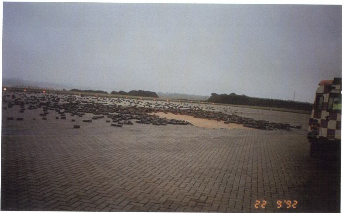
FIG 1. DAMAGE TO THE RUNWAY THRESHOLD TURNING CIRCLE
